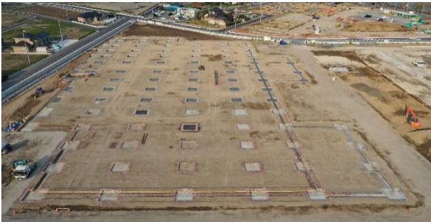
Fig. 3. Example of a construction site of TNF system (at the stage of completion of footings).
